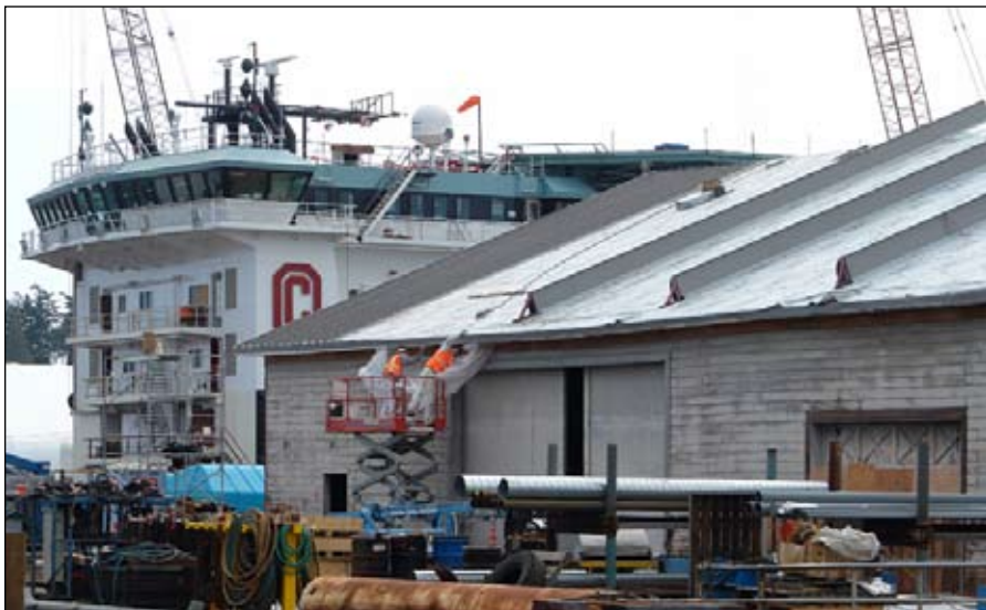
Contractors (orange vests) work on installation of a new roof on historic Port of Anacortes Warehouse 4, adjacent to the Dakota Creek Industries (DCI) shipyard.
