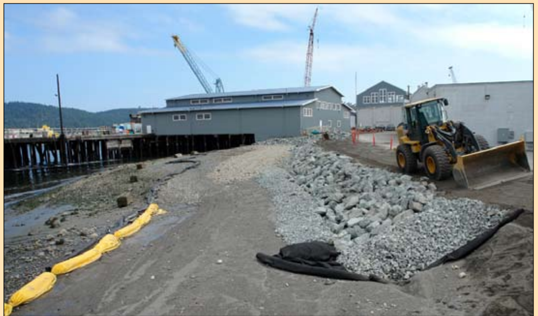
BEACH PROJECT: Those familiar with this stretch of beach near the main Port Warehouse will notice improvements including removal of old creosote pilings and concrete rubble.
