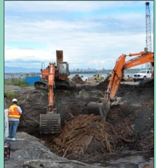
Clean-up of the former Scott Paper mill site continues on several fronts near downtown Anacortes on the Fidalgo Bay shoreline. While crews continue to dredge/cap and construct new breakwaters, others are engaged in upland remediation. Contaminated materials from the site above will be removed and disposed of before new fill is added.
