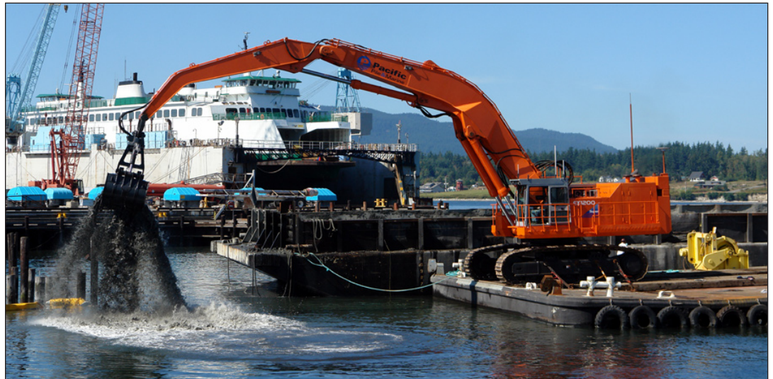
Crews contracted by Dakota Creek Industries continue dredging at the shipyard site on the Guemes Channel.
